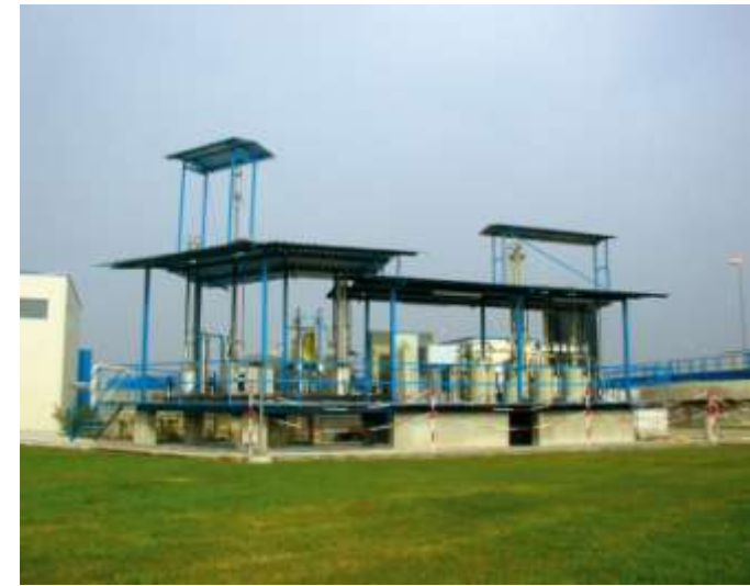
Biogas treatment plant in Murcia Este WWTP
